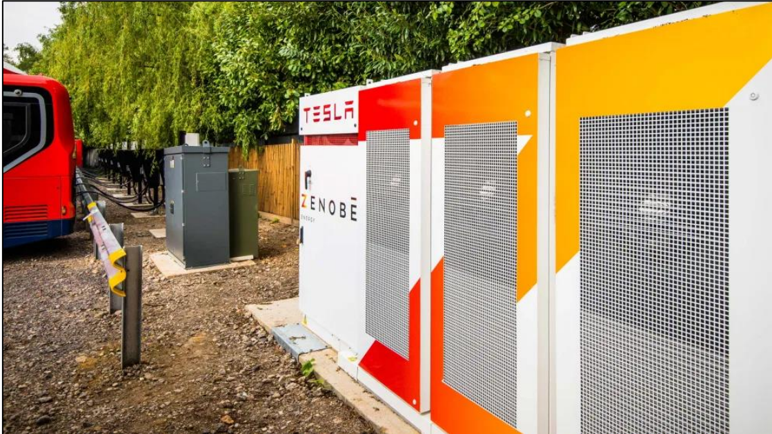
Figure C-3: Tesla Powerpack (78 units) installed at Stagecoach's Guildford Dept
